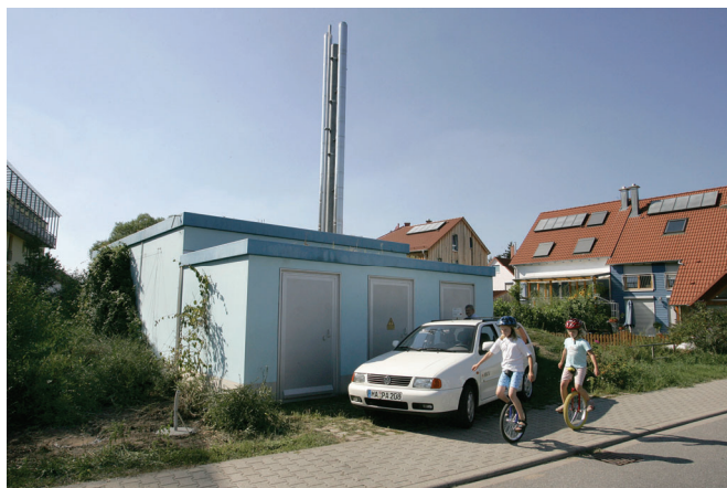
Figure 3: The low voltage grid segment “Am Steinweg” is connected to the medium voltage grid via the transformer in this building. The combined heat and power plant is integrated into the same building at the rear side. (Source: MVV Energie)
