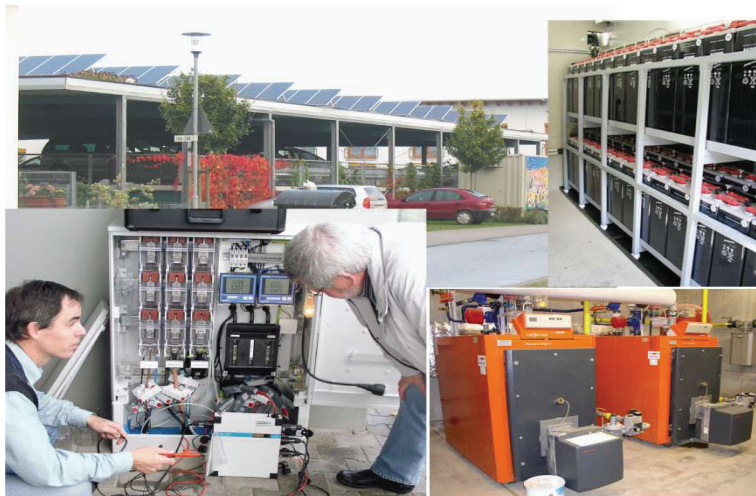
Figure 4: Pilot installation "Am Steinweg", Stutensee (Germany), operated by MVV Energie AG.
